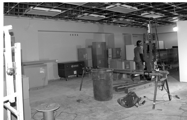
THE ISIS HMC FACILITY WILL HOUSE A FULLY-OUTFITTED 8 STATION WET-LAB.
